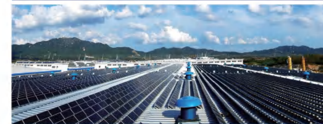
Solar panels arrays
